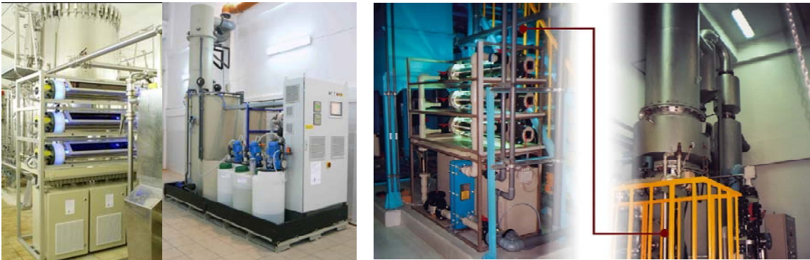
Photo 1: Left side is a Pharmaceutical application (Antibiotics and X-ray waste) Middle is in metal industry (cyanide detoxification, Phosphite –Ortho Phosphate oxidation and oil emulsions sequential treatment) Right side: combination of gas washing and UV treatment, without residue
