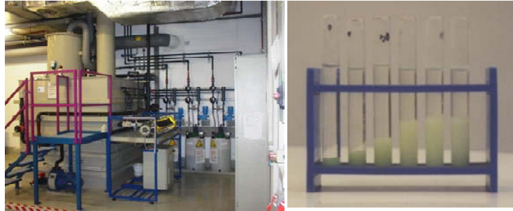
Photo 2: left the treatment plant for the detoxification of Cu EDTA at Multek, completely delivered and installed by a.c.k. aqua concept, the inventor of the Enviolet®-technology
